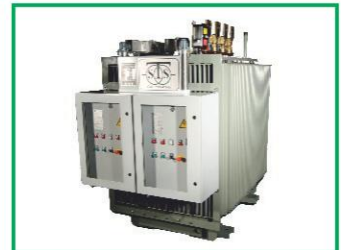
3150 kVA, Multi-tap Test Transformer with motor drive tap-changer installed in U.S.A
